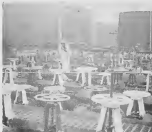
Trickiest part of the refueling job is lining up the pipes to carry the oil from tank to ship. Out of this maze of pipes and valves the operator selects the correct ones that lead to the Kosmos III. After the "manifold" is set up, the lines are checked to see that they are full.
